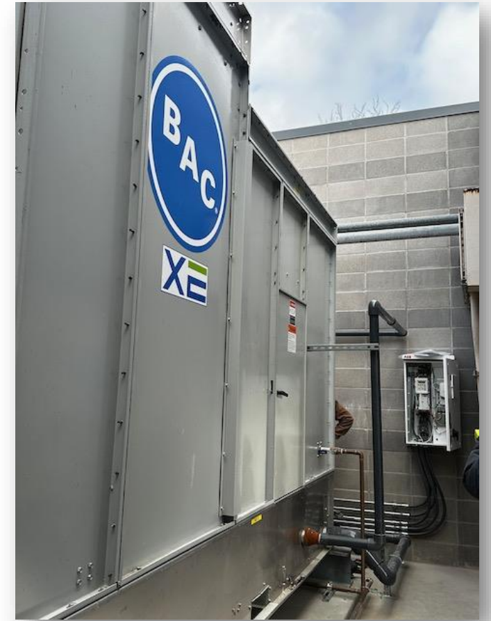
New Cooling Tower
